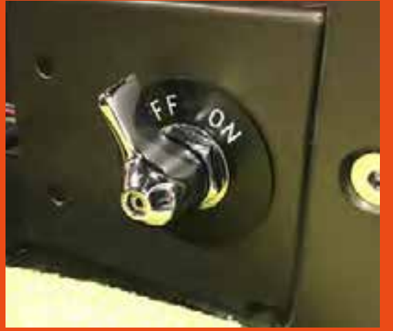
Battery cut off switch on driver's side seat riser We had the On/Off bezel engraved with typeface that matches the typeface used on the gauges and the switch panel.
