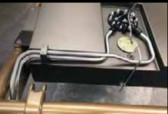
Stainless fuel tank installation along with stainless plumbing.
