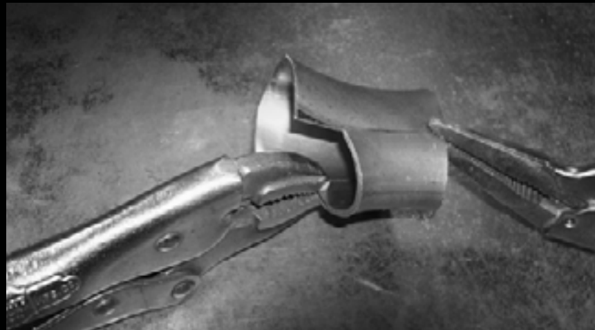
Small pieces of exhaust tubing were squeezed in a vise to get their oblong shapes and welded together to create the base of the standoff.
